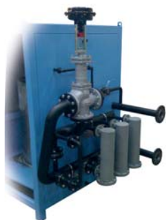
3 channel valve on cooling circuit
