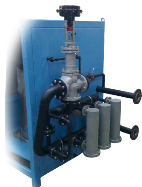
3 channel valve on cooling circuit
