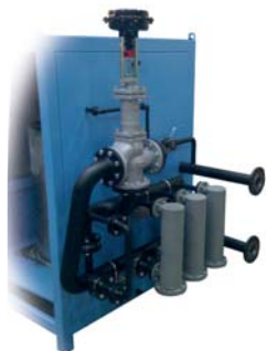
3 channel valve on cooling circuit
